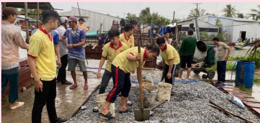
Civil Engineering students applied their professional knowledge to support local people in building bridges and roads.
